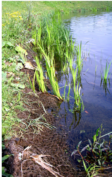
Fig. 3. Bank of the restored water reservoir stabilised with coir rollers with cultivated vegetation. Photo L. BERAN.
